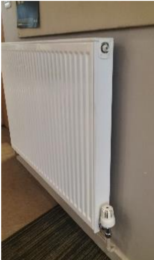
Radiator in communal kitchen area in the flat. This also has an adjustable radiator valve.
