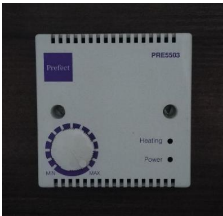
Thermostat in some of the rooms in St Johns Halls.
