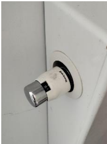
Radiator in corridor showing a frost symbol on valve.
