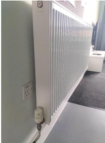
Radiator showing temperature valve in common area in flat.
