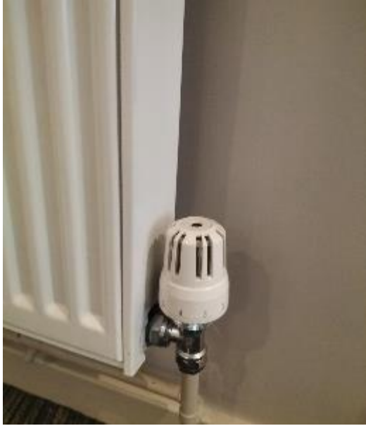
Radiator valve. Turn this left or right to adjust the temperature up or down.
